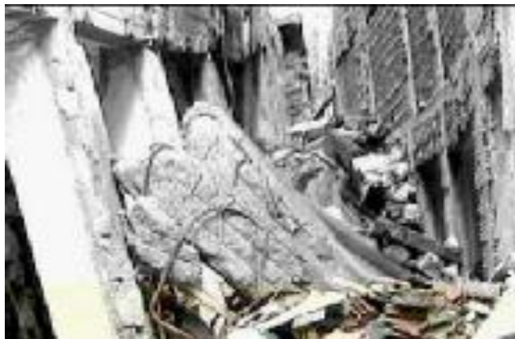
Fig: Damage of Izmit earthquake. [Source- Mizan Dogan]
