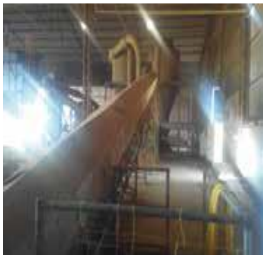
Picture 5: Conveyor Unit
