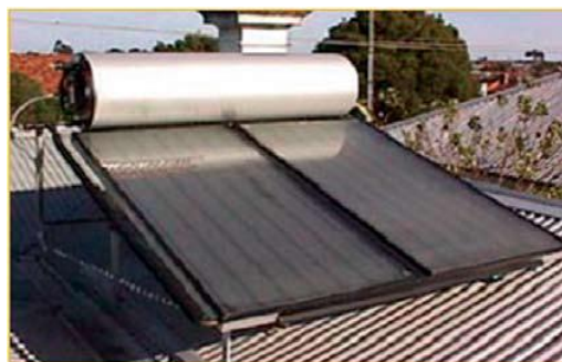
Solar Domestic Hot Water (Thermo siphon) System
